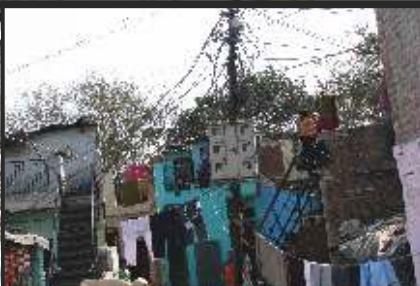
This utility pole in Tigri has numerous unauthorised taps, which are dangerous and often lead to electrocutions.
